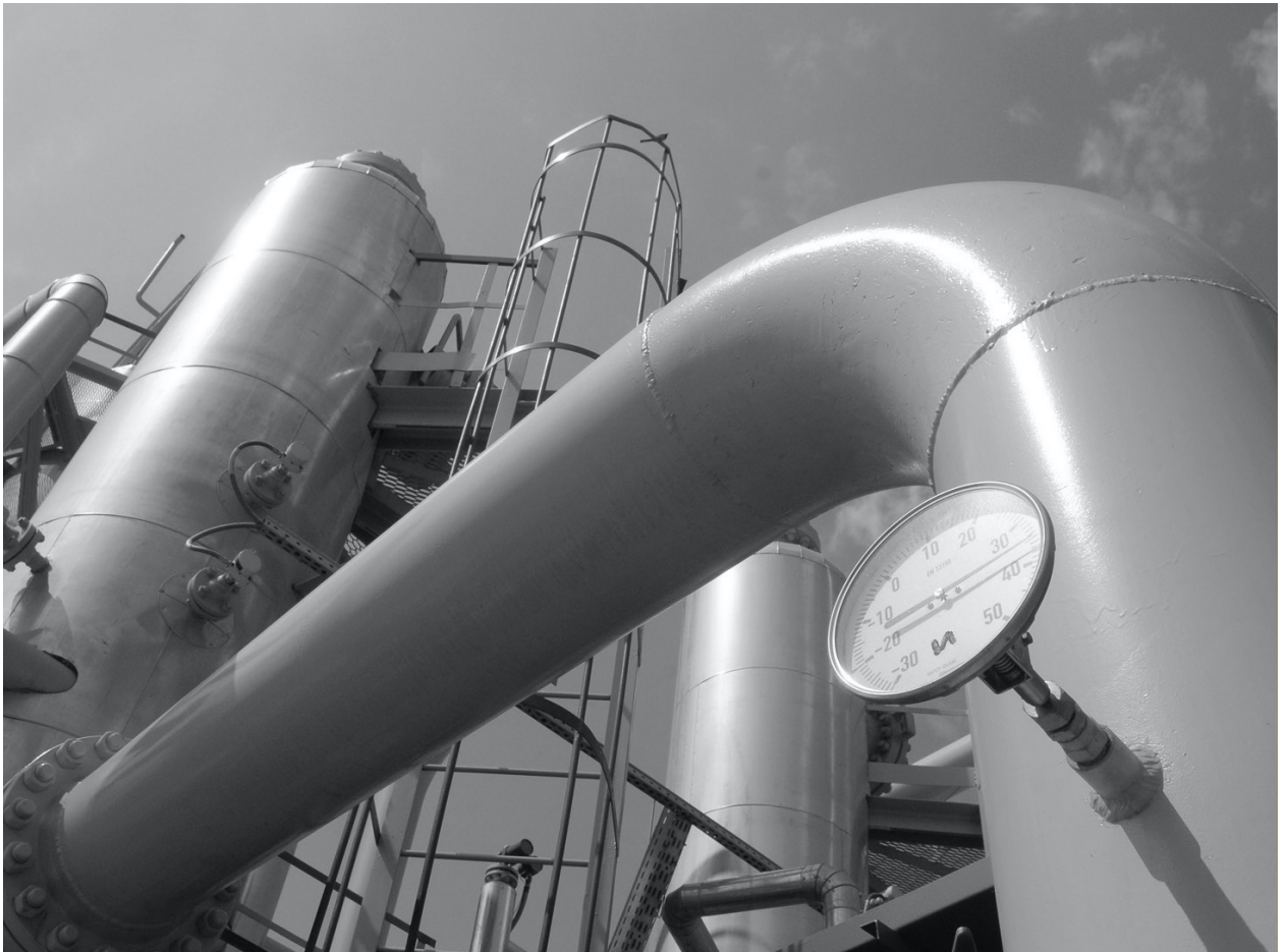
► Fossil gas compressor station
